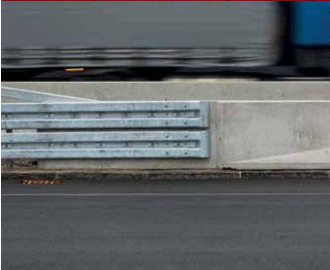
BELOW: Focus is shifting to the transition points where one system joins another.
